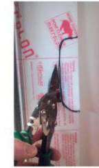
Step 4 – Mark and cut closure strips to fit around handrail, etc. using tin snips. Closure strips may be bent by hand or with duck bill pliers. Lap strips to make an air tight seal.
