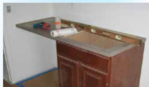
PREVENT COUNTER TOP & CABINET DAMAGE
